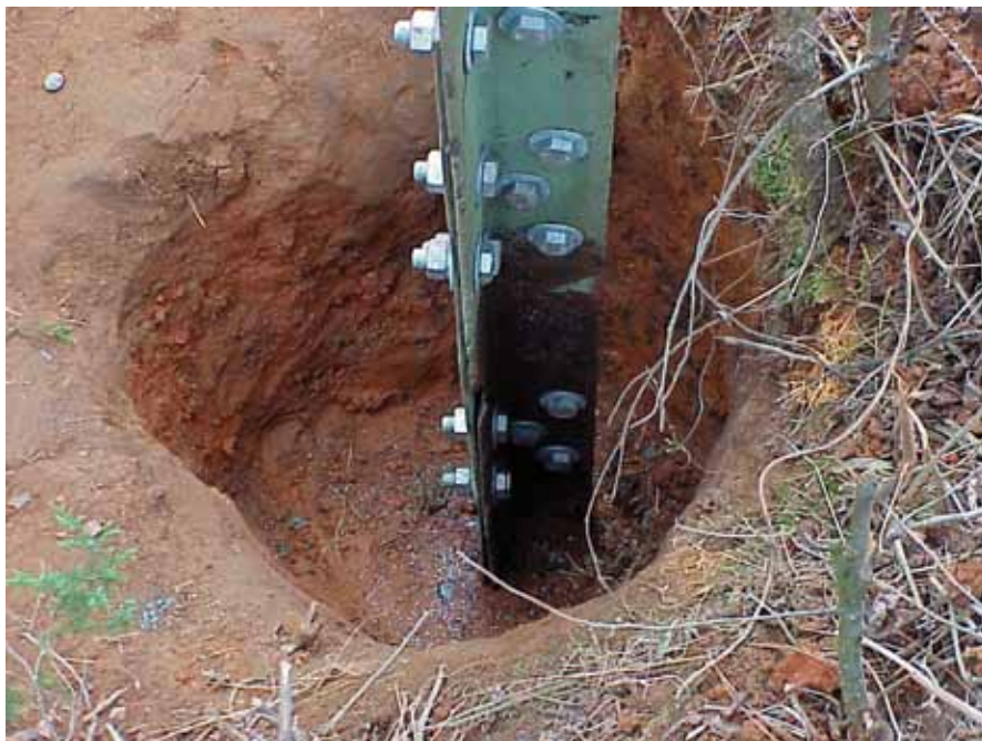
A recently repaired embedded steel footing is shown. Photo courtesy of Alan Holloman, Georgia Power Co.
