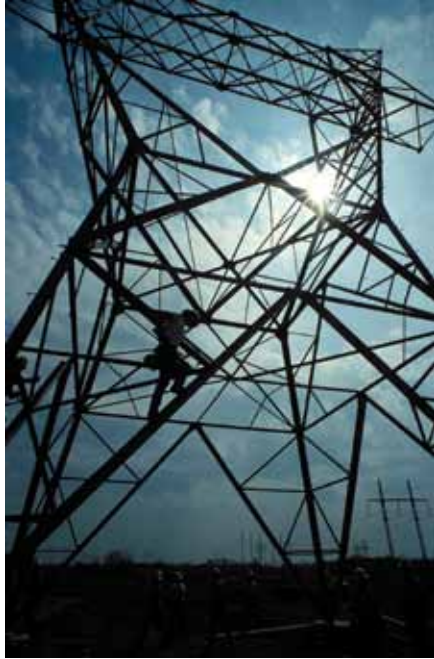
Workers conduct a final inspection of a newly installed galvanized steel transmission tower. Photo courtesy of Alan Holloman, Georgia Power Co.
